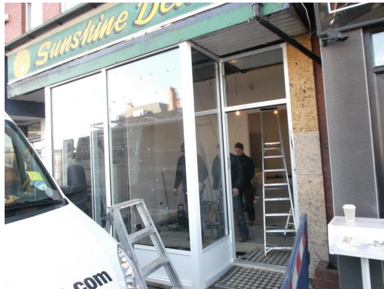
Poorly designed new shopfront - after
